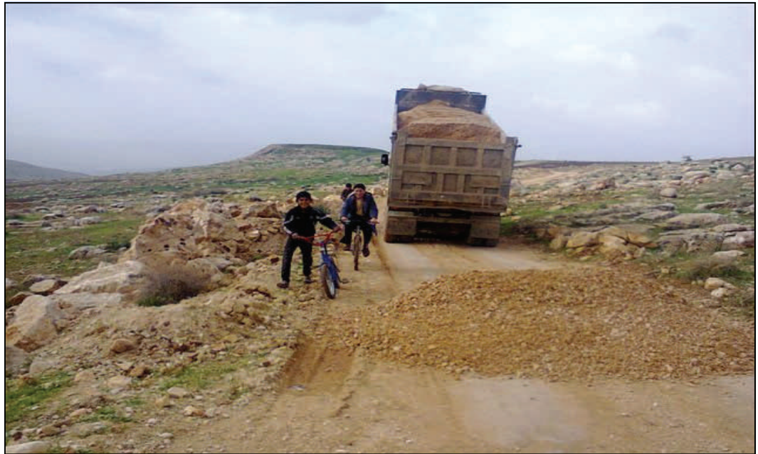
Rehabilitating roads in northern West Bank as part of improving access to water.
